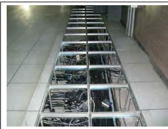
Raised flooring with obsolete wiring (2006)
