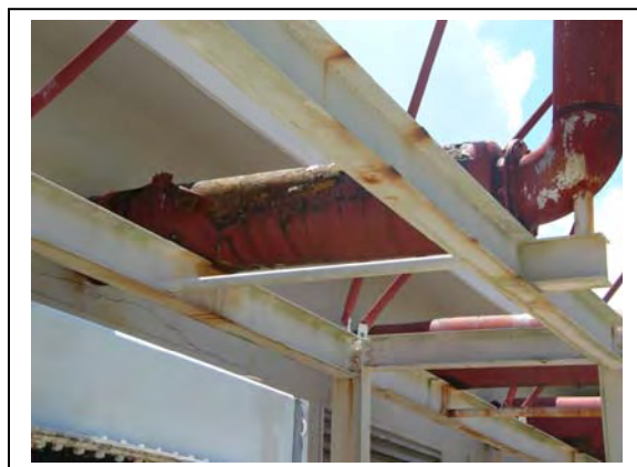
Corrosion of roof top exhaust vents (2006)
