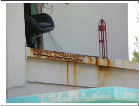
Exposed reinforcing bar, spawling concrete and loss of metal railings. (2006)
