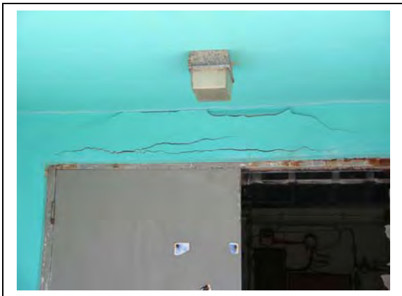
Lintel cracking above ground floor entrance (2006)
