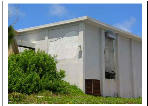
Radar building. Southern facade with notable damage to ventilators, stucco finish, corrosion of all metal. (2006)
