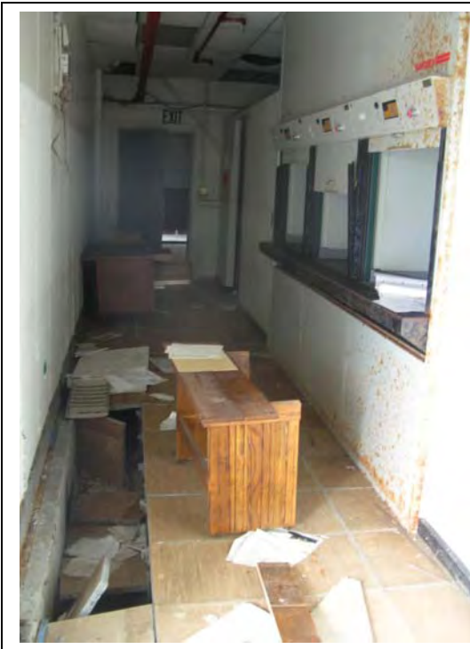
Typical damage to raised floor and corrosion of all interior finishes (2006)
