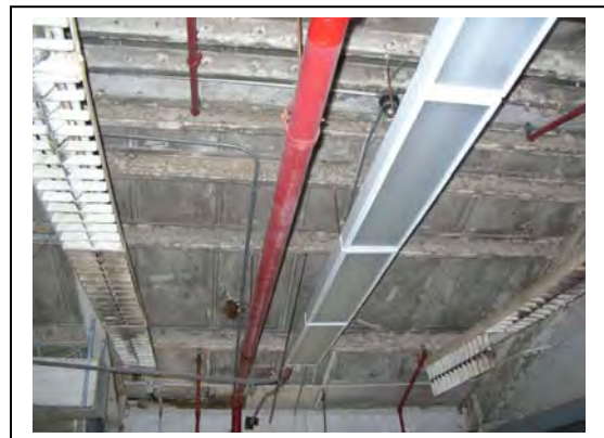
Corrosion of beams & spawling of roof (2006)
