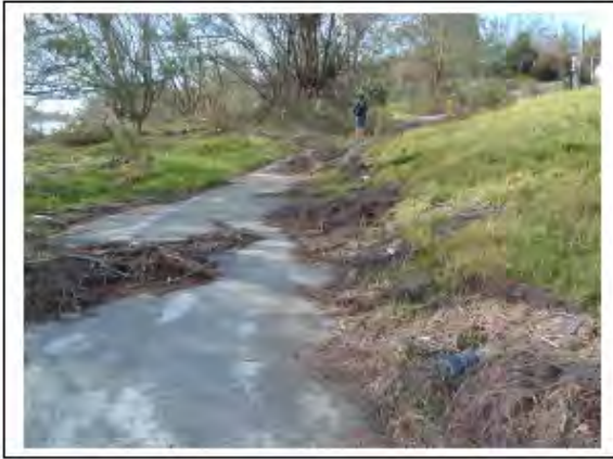
1. View from gate showing storm surge over main access road into Cooper's island
