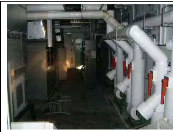
Utility room with little visible damage (2006)
