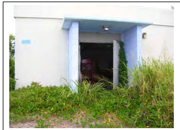
Pumping station in neglected state (2006)
