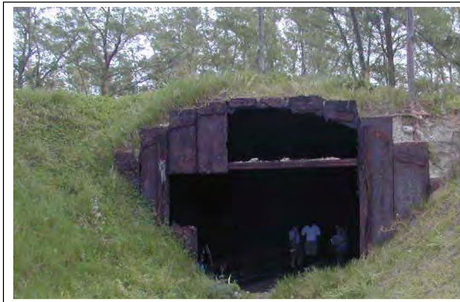
Figure 27: Bunker in dangerous state of disrepair.
