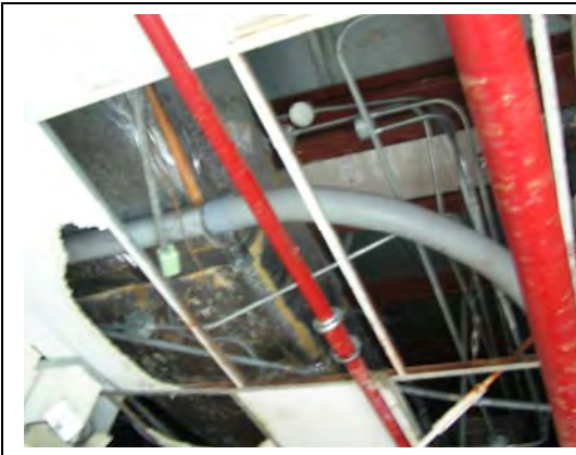
Damage to suspended ceiling (2006)
