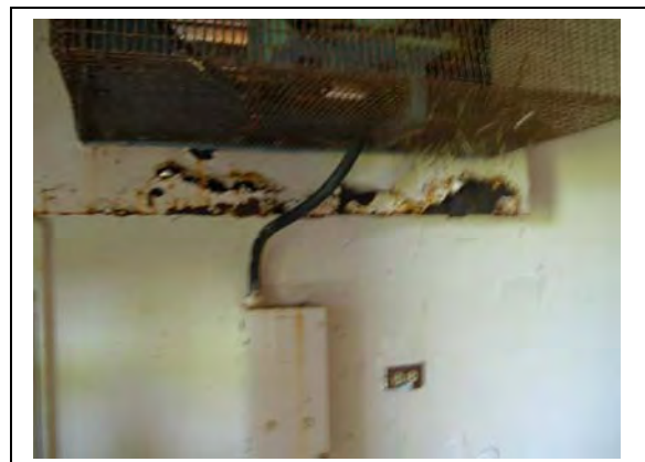
Corrosion of HVAC systems (2006)
