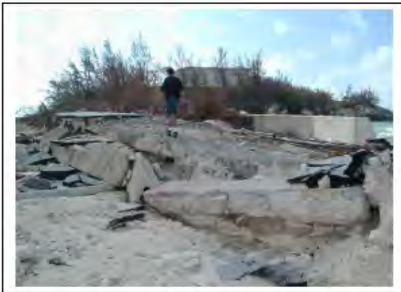
4. View to outer island showing bridge link completely destroyed.
