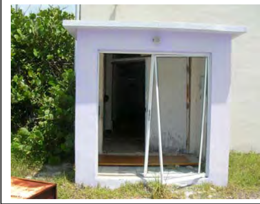
T&C building entrance recently broken open (2006)
