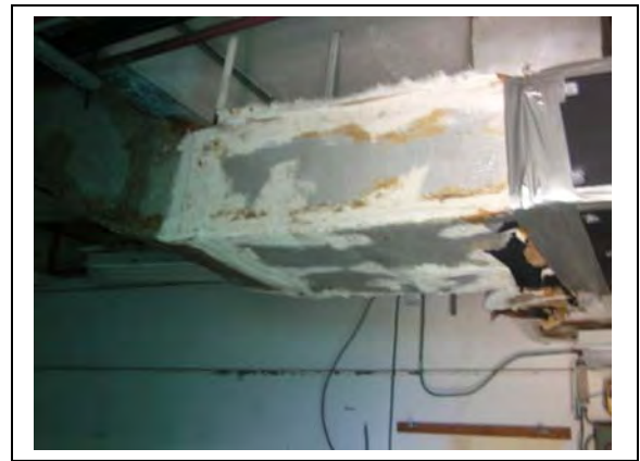
Corrosion of HVAC systems. Also noted that the duct systems are repaired with duct tape and plywood (2006)
