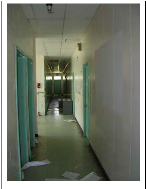
Corridor with limited physical damage. However the centre has been broken open and some minor vandalism has taken place (2006).
