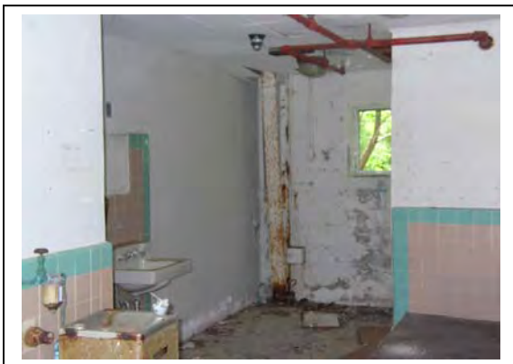
Bathroom with extensive damage (2006)
